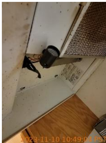
Hood Bulb Missing
