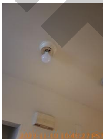
Light Cover Missing 📅 2023-11-10 12:45:27
