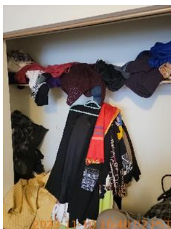
Closet doors missing 📅 2023-11-10 12:40:02
