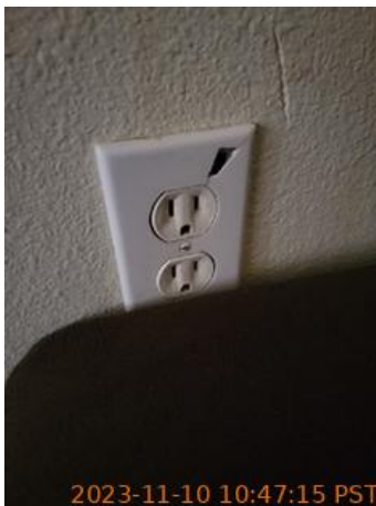
Broken Outlet Cover
