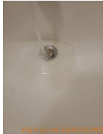
Sink Slow Drain 📅 2023-11-10 12:43:55
