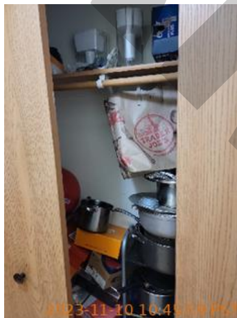
Closet Doors Not Functioning
